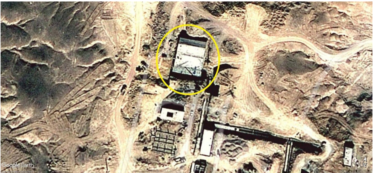
The imagery of the 2009 Semnan site after the start of the construction of concrete foundations
