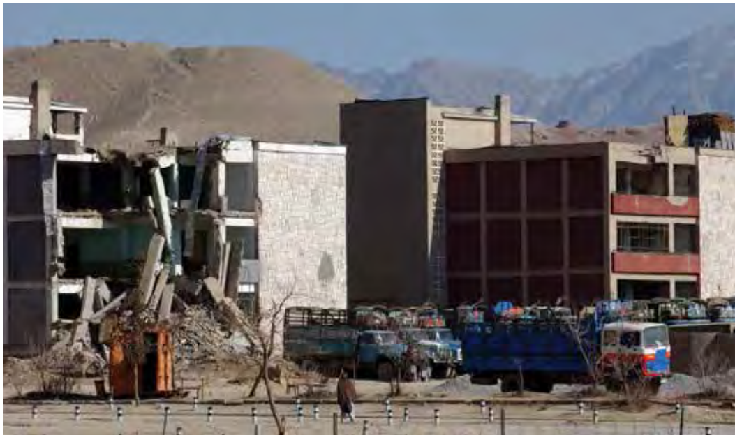
Damaged infrastructure at KMTC in Kabul that needed to be repaired before basic infantry training for new Afghan recruits could start. (Photo by Jason Howk)
